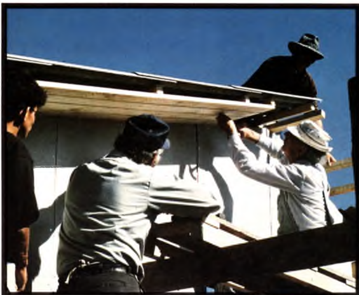
(Diagonally, l. to r.) Rev. Self (lower right) works on a cornice at a church in San Antonio, Chile.
