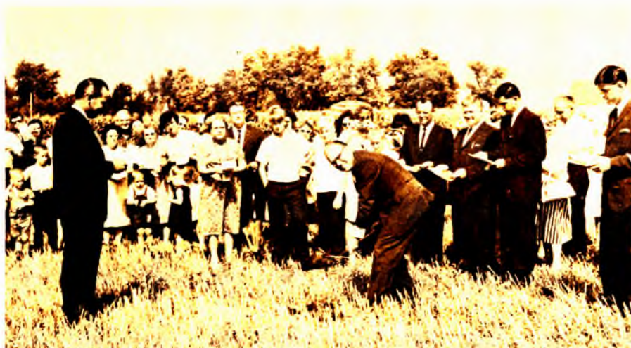
Ground breaking for the new Crystal Lawns Church in Joliet. At the left is Rev. Lawrence Jantz, pastor of Joliet First Church. Dr. Mark R. Moore, district superintendent of the Chicago Central District, turns over a shovelful of dirt. Behind him are Earl Summers, chairman of the board of trustees; Vern Bond, chairman of church building committee; Rev. Lynn Smith, assistant pastor; and Wayne Frankhauser, N.Y.P.S. president.
